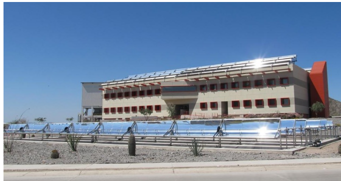
Solar Concentrator Chiller System, HOLCIM Mexico 2010-12
